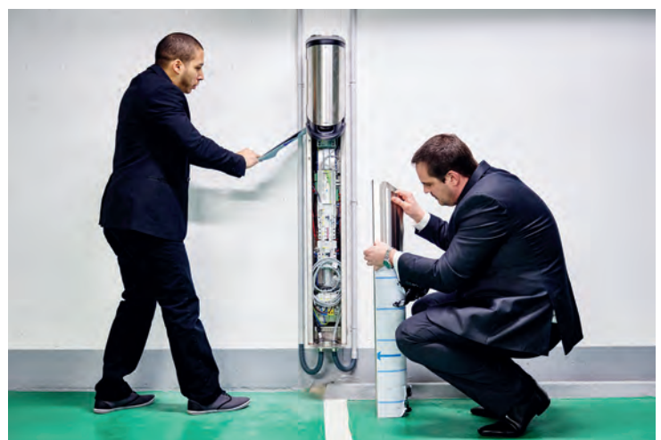
All poles were in place, and Project Manager Jonathan Velmy (left), together with Ensto Sales Manager Jérôme Perdu , peeled the protective plastic from the stainless steel poles.
